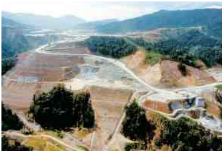
The Batu Hijau copper and gold mine passed completion tests in October 2000 and is now in full operation.
