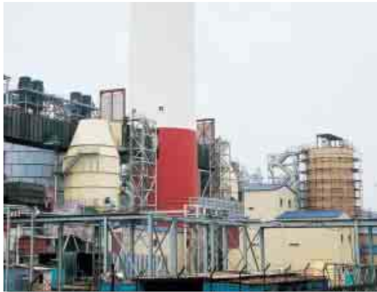
Coal-fired thermal power station we are constructing in Vietnam through a partnership with manufacturers in Korea, the U.S., the U.K., and Australia.
