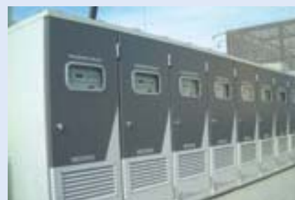
The micro gas turbine co-generation system installed at a hospital in Kyushu.
