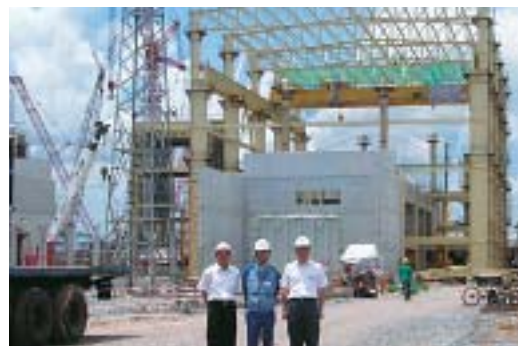
Construction site at the Phu My 2-2 thermal power plant, the first independent power producer in Vietnam
