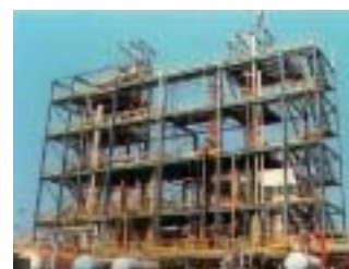
Facility in India to destroy Hydrofluorocarbon (HFC23)
