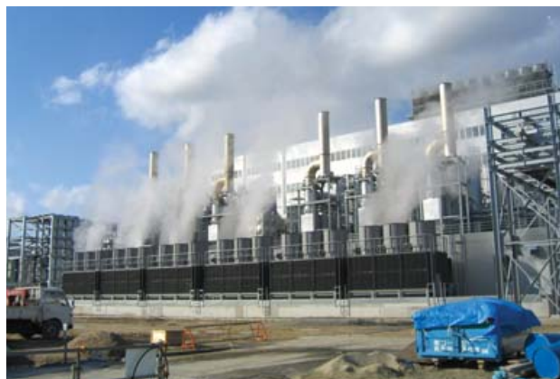
We established SC Hiroshima Energy Corporation to provide energy services to Hiroshima Elpida Memory, Inc. Equipped with a gas engine cogeneration system (33MW) fueled by natural gas, we will provide electricity and heat for the next 15 years.
