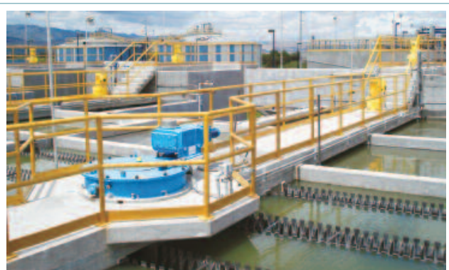
The San Luis Potosi Wastewater Treatment Plant we operate in Mexico
