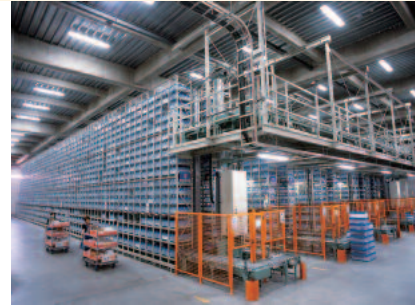
Automated distribution center
