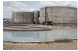
Greenhouse gas reduction project through collection and utilization of methane gas from wastewater from a tapioca flour plant (Indonesia)
