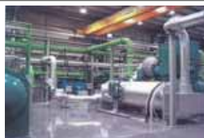
Energy-saving type district cooling project (UAE)
