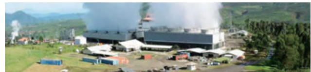
Wayang Windu Geothermal Power Station in Indonesia
