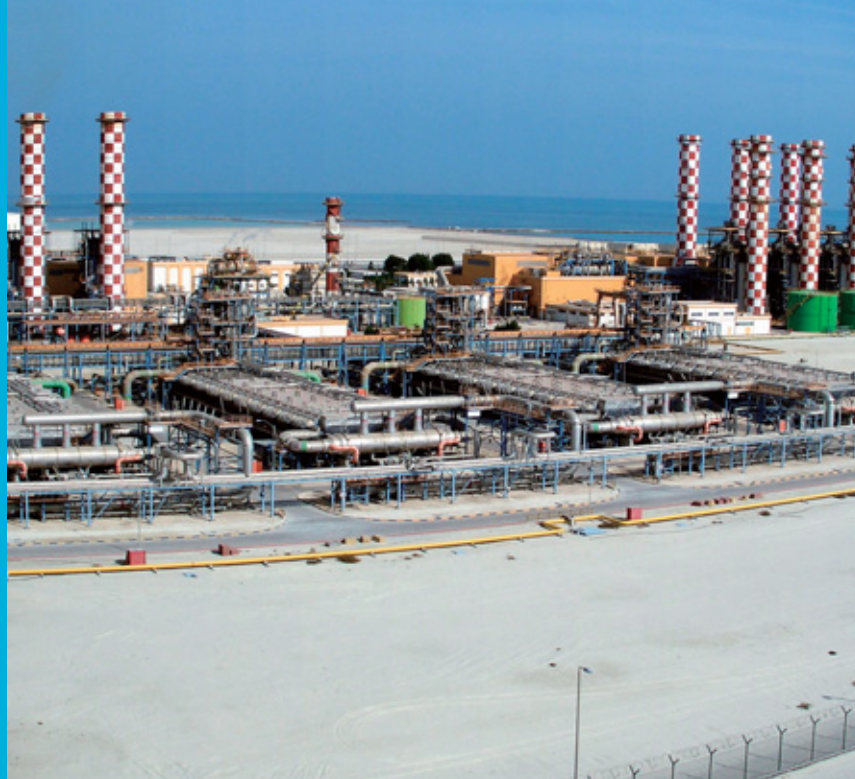
Our Al Hidd power generation and desalination project in Bahrain, the first privately managed power and water project in the country (approx. 1,000 MW of power generated and daily 405,000 tons of water treated)
