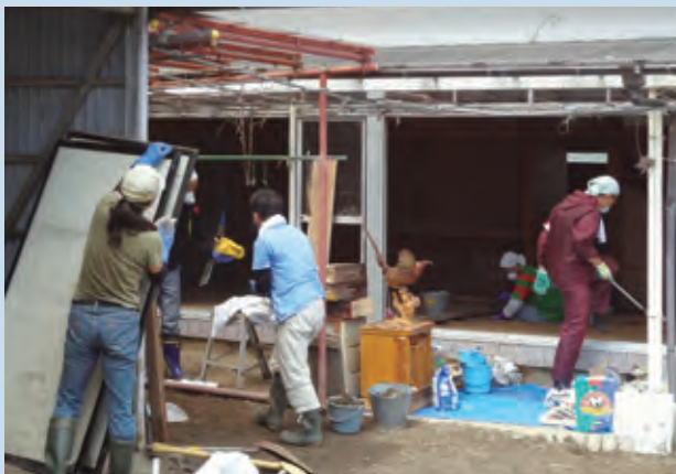
Removing debris and mud from houses
